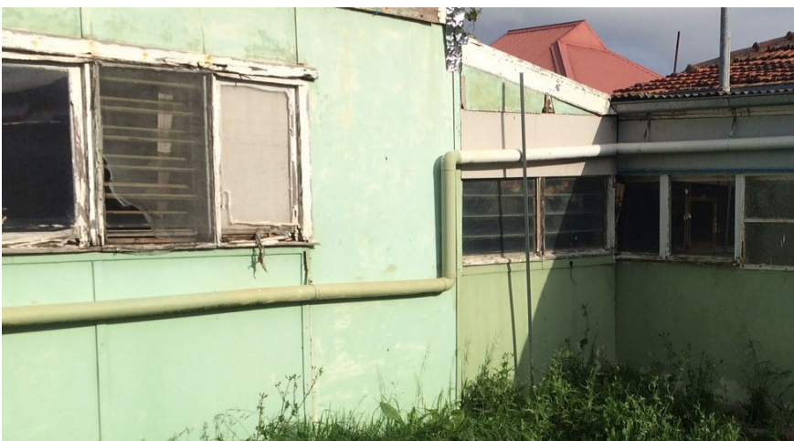
Minimum rental standards would help to bring properties like this Footscray home to a basic, liveable standard.
