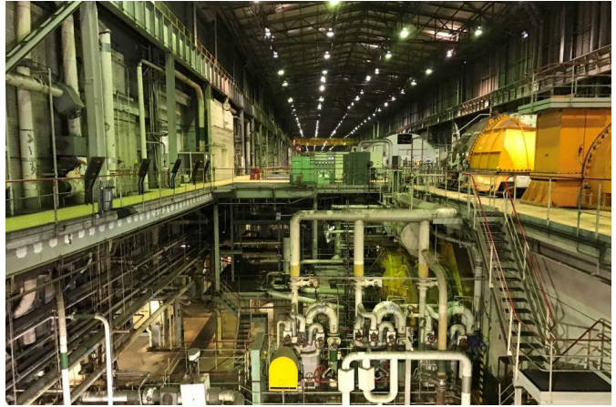
Figure 16 Hazelwood Power Station generator room. Source: ABC.
