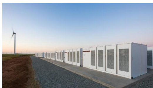
Figure 26 Hornsdale Power Reserve
