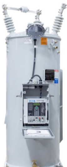
Figure 24 – Example of an Overhead Voltage Regulator
